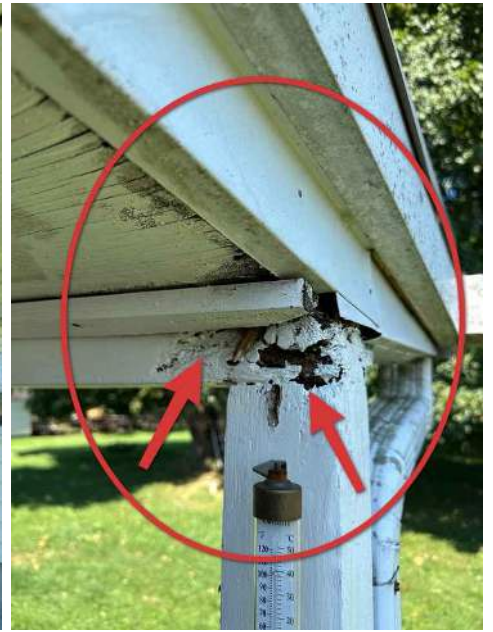
Rotten post and carrier beam
