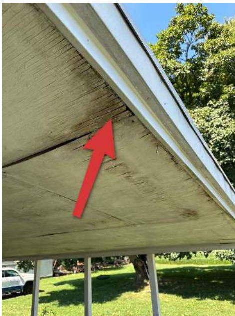
Rotten porch ceiling plywood
