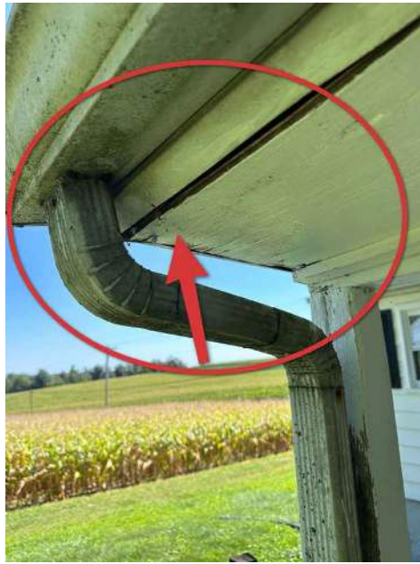
Softening soffit member
