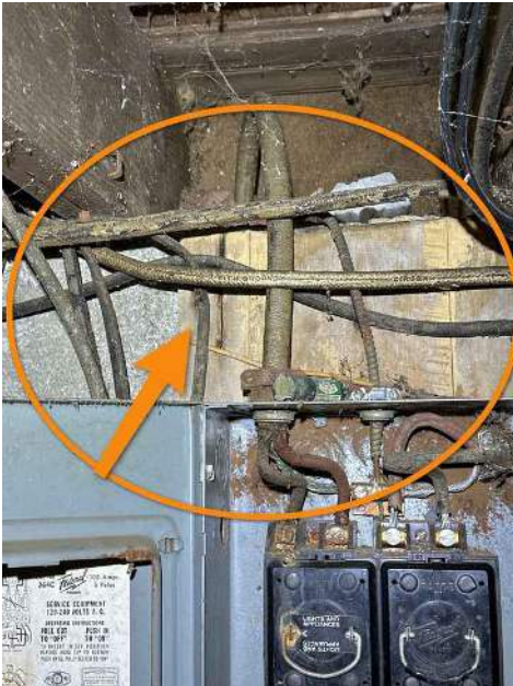
Representative of wiring Throughout
