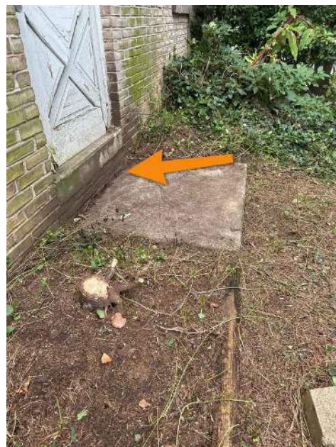
Settling back towards garage
