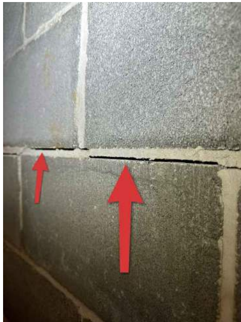
Left side horizontal crack
