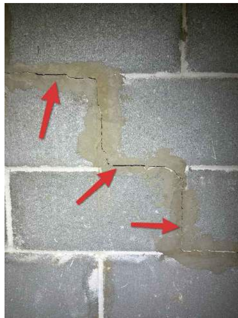
Front Foundation Wall Step Crack
