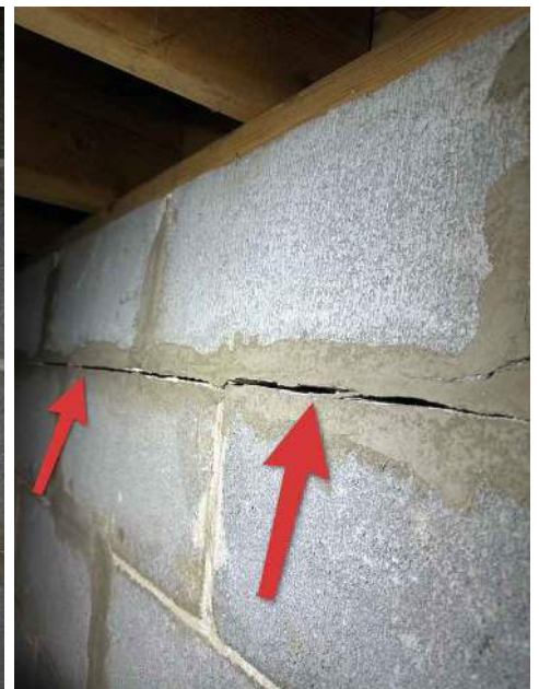
Foundation Wall Horizontal Crack
