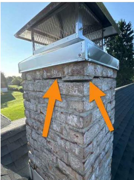
Close up - bricks lifted opening up mortar joint
