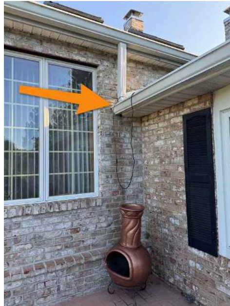
Recommend flashing to divert water into gutter
