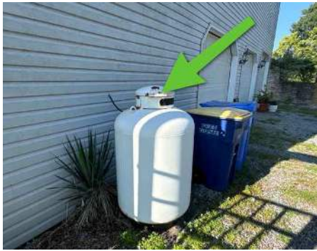
Propane shut off
