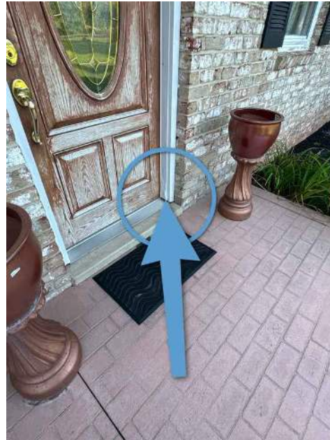
Wood under vinyl rotted
