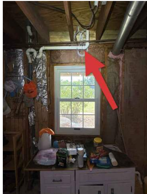
Water dripping from drain line
