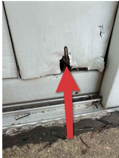
Wood rotting behind vinyl
