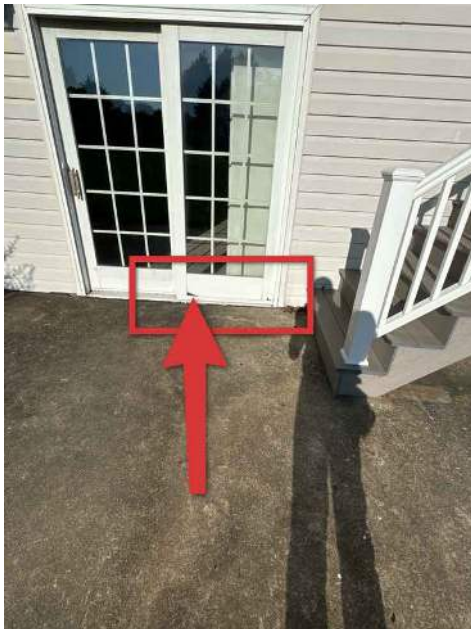
Base of door rotted
