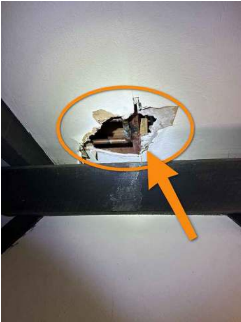
Possible mold in ceiling
