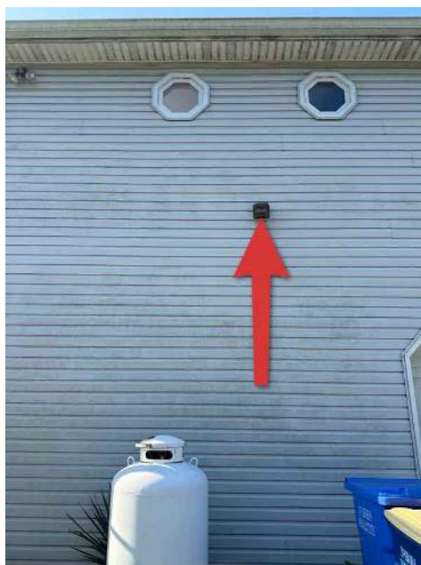
Lint clogging vent
