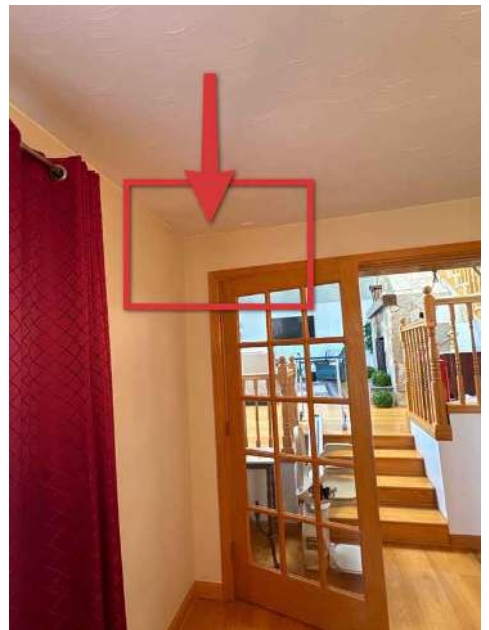
Corner of wall and ceiling wet
