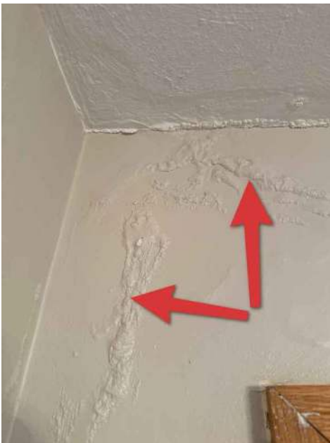
Close-up of blistering
