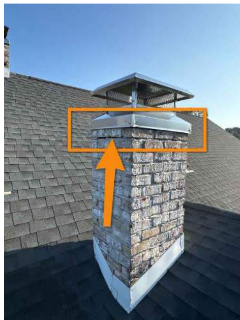
Upper layers of brick gapping and loose
