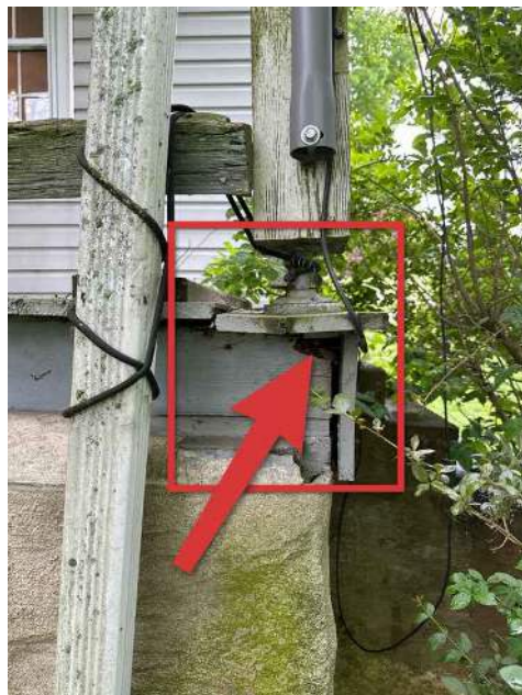
Post settlement due to rot
