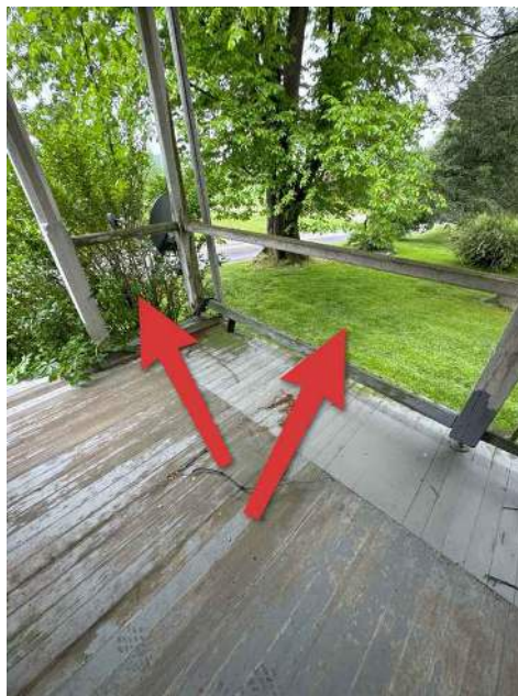
Railing balusters missing
