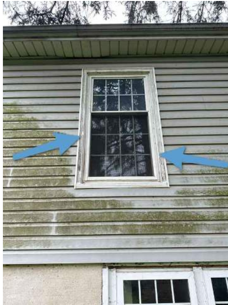
Peeling paint on some windows
