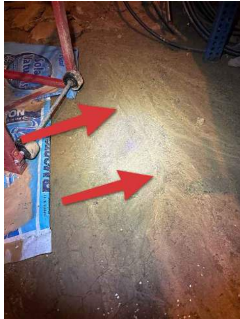
Mudflow across floor
