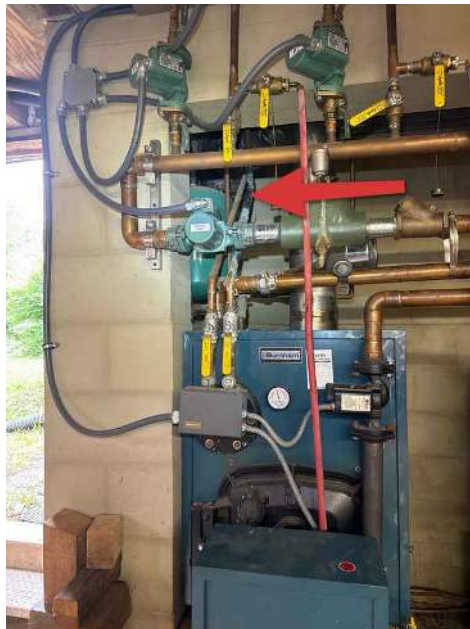
Domestic line leaking
