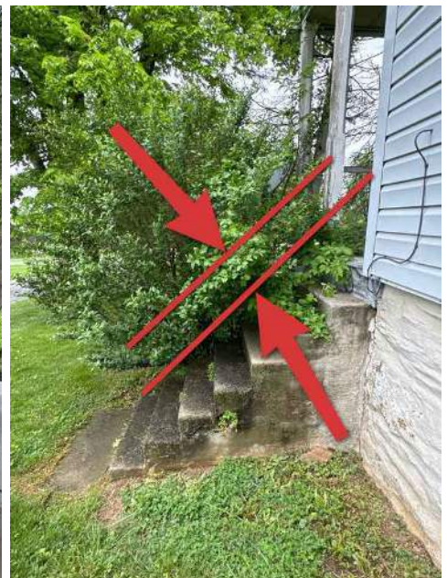
Stair railings and balusters missing
