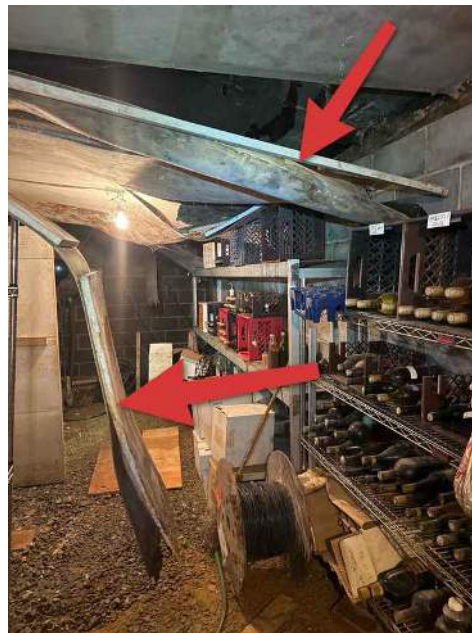
Insulation panels falling down
