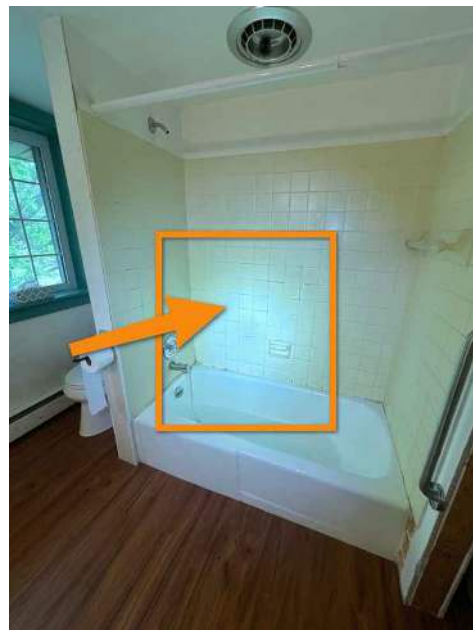
Grout repair needed
