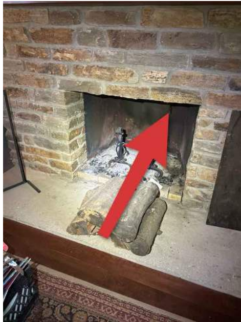
Damper not working
