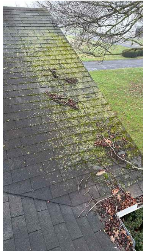
Excessive biological growth
