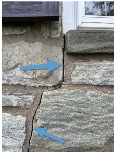
Crack in stone veneer joint
