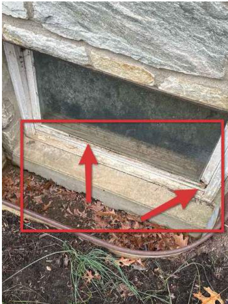
Rotten sash basement window
