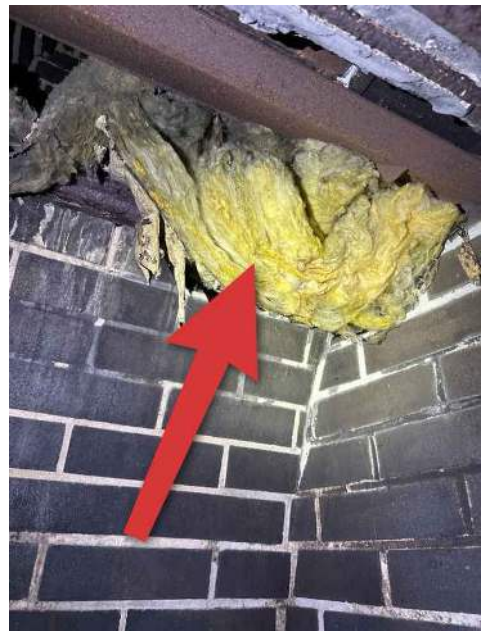
Insulation blocking flue Basement
