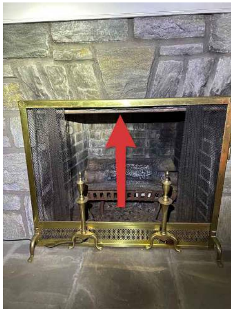
Flue blocked Living Room
