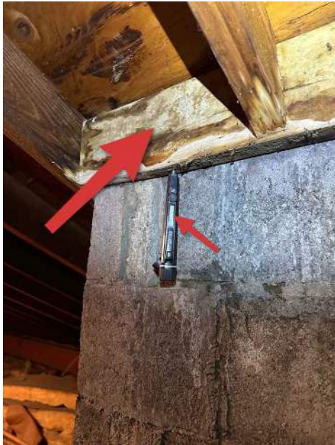
High moisture reading at framing
