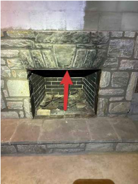
Basement flue blocked
