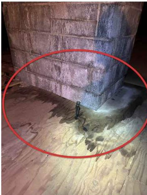
High moisture at floor
