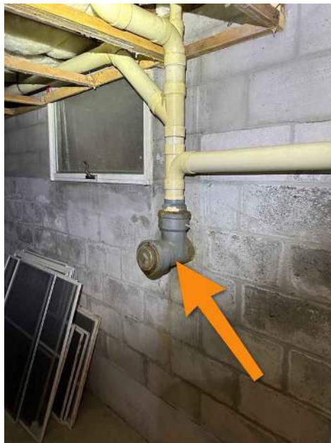
To septic system
