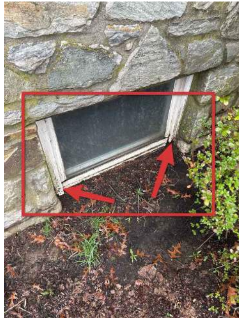
Rear Basement Window rotten
