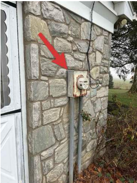
Pulling away from wall
