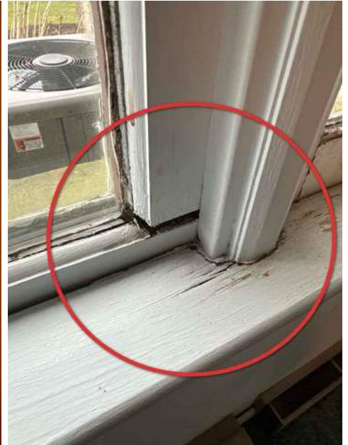
Rotten sash and sill Dining Room
