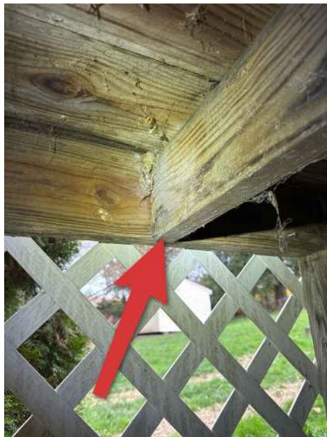
Joist hangers missing at rim joist
