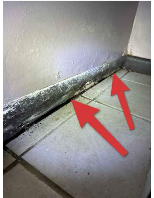
Moisture soaking through trim
