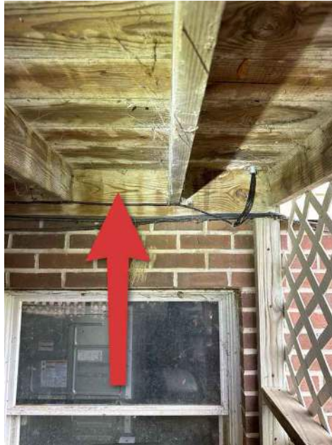
Lateral load connectors missing
