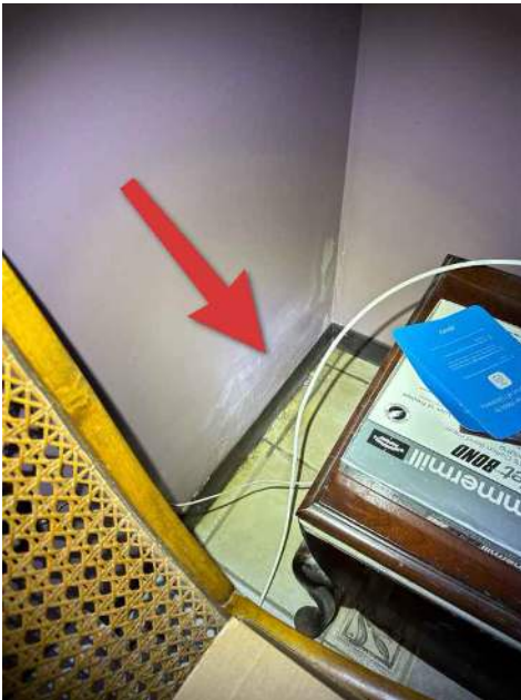
Moisture, extending into adjacent room
