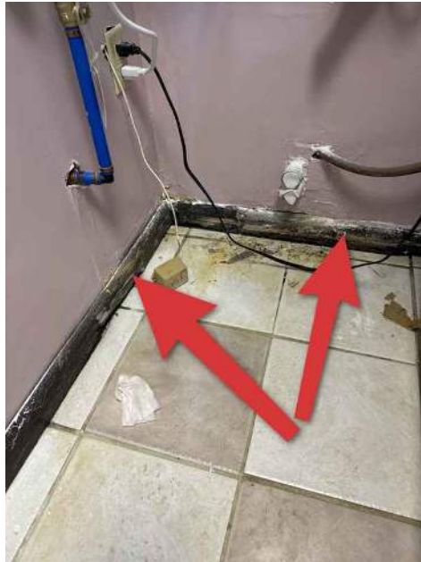
Moisture at base of wall
