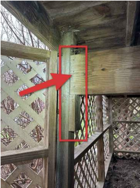
Beam support not adequate
