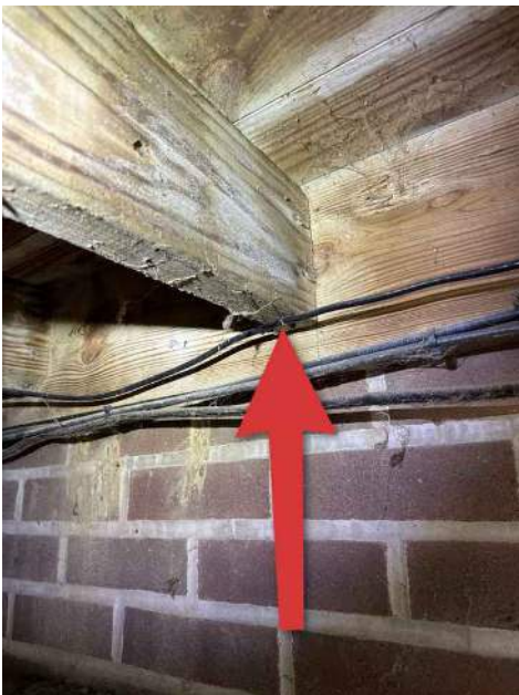
Joist hangers missing at house
