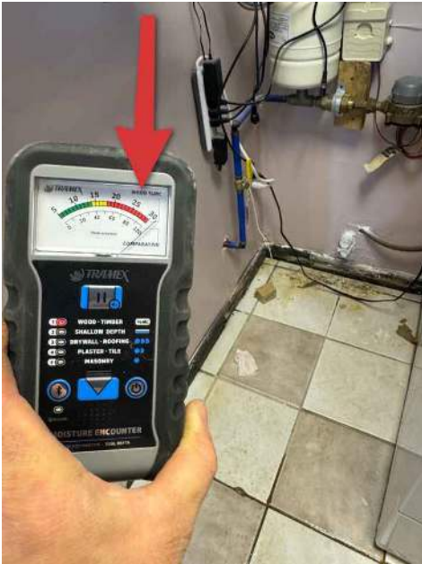
Wet reading on meter
