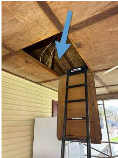
Moisture stain in corner of roof valley
