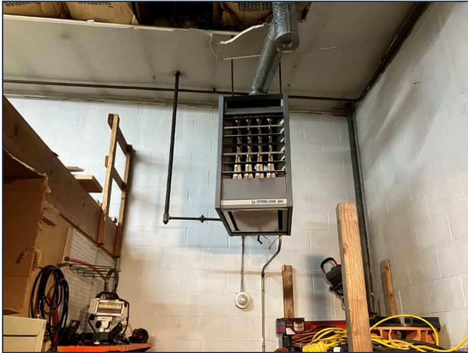
Natural gas heating unit in 5-bay garage
