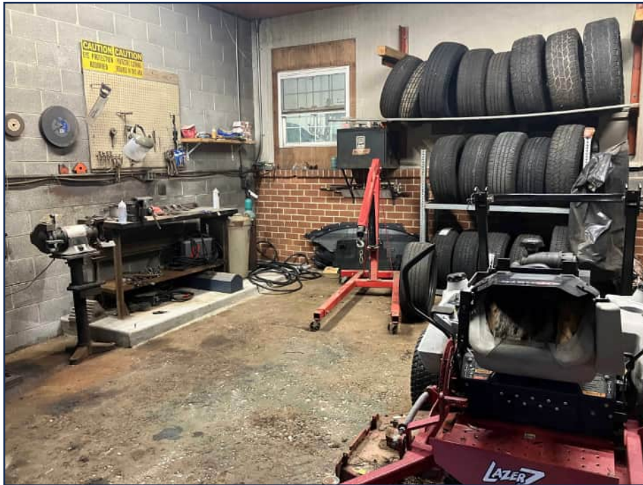
De minimis staining in maintenance building
