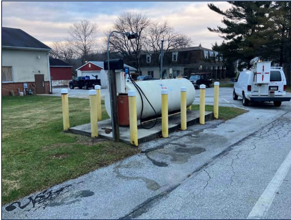
1,000-gallon diesel fuel AST with dispenser
