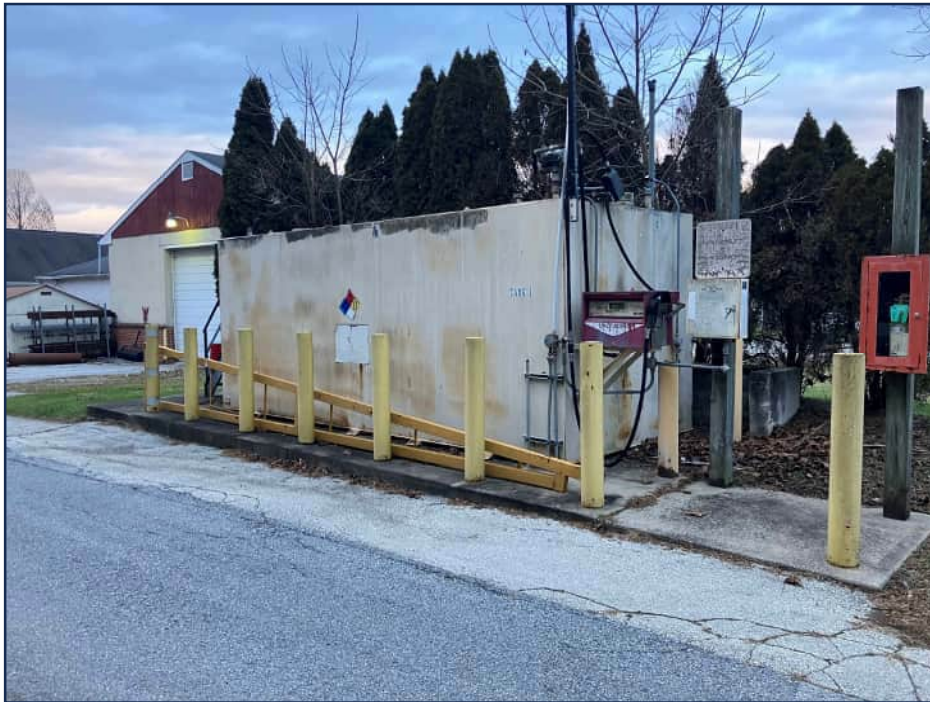
6,000-gallon gasoline AST with dispenser
