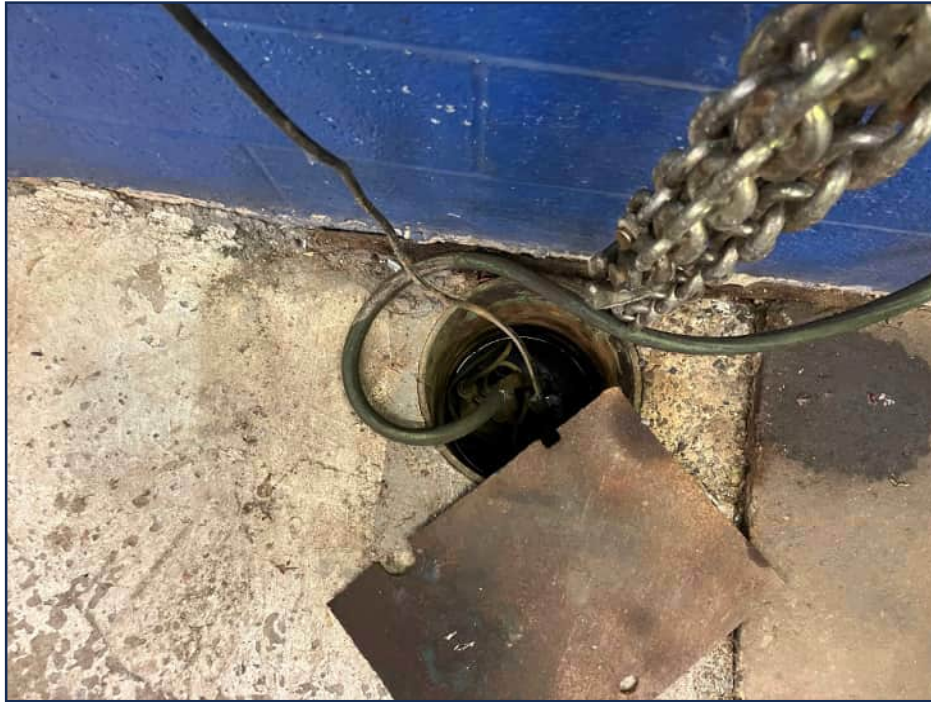
Sump and discharge hose in maintenance building
