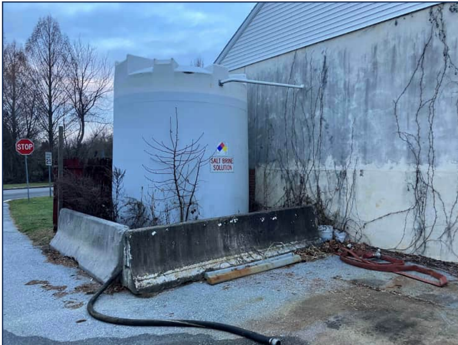
Brine tank outside of 5-bay garage
