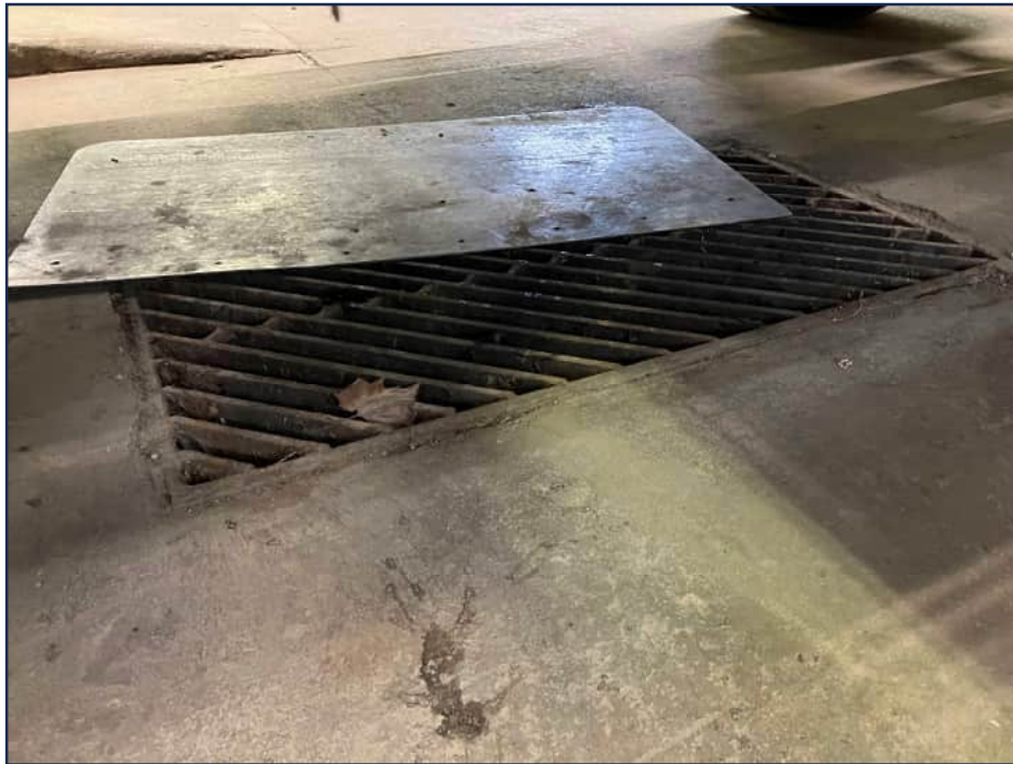
Floor drain in maintenance building
